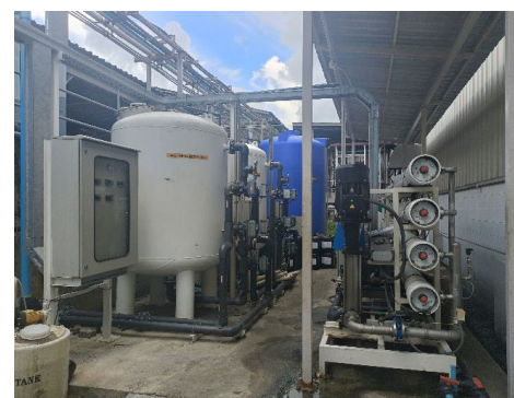
SATL's water recycling equipment
