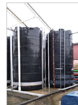
SMM's rainwater tanks
